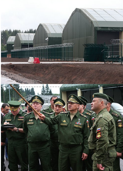
Russian Ministry of Defense photos from Defense Minister Sergei Shulgo's visit to the 26th Missile Brigade at Luga in June 2014 show unique tent-garages under construction for Iskander launchers.
